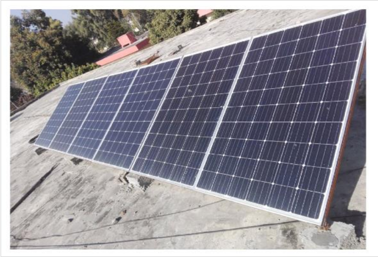
Figure 22 PV Installation on the rooftop
