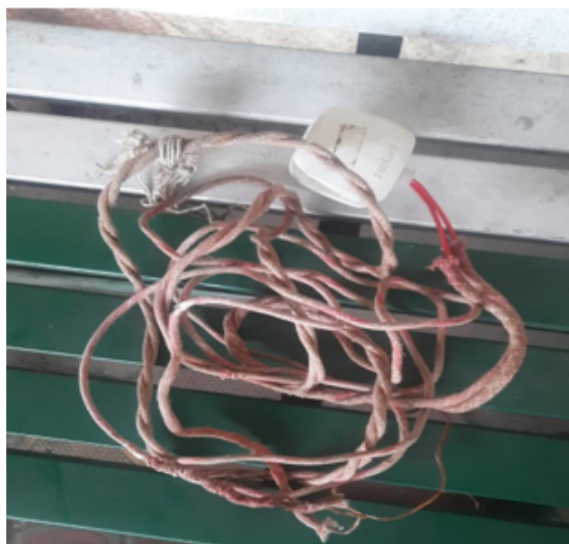
Fig. 2: Photo of disconnected electric wire having uninsulated ends.
