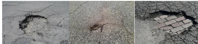
Figure 1. Road image(s) with Pothole [1]
