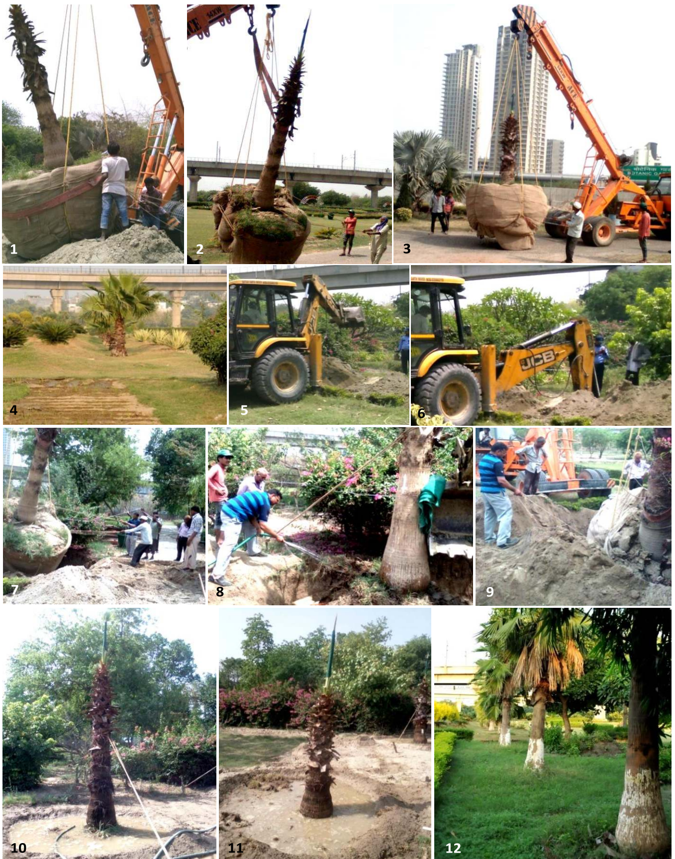
Photo Plate IV: 1. Root ball after lifting was kept on ground to move further, 2. and 3. Trees on the way to new location, 4. Transplantation site, 5. and 6. Mechanically digging is in progress, 7. Process of placement of root ball in pit/trench in right position, 8. After resting root ball properly in prepared pit, extensively watered, 9. To make transplanted tree stable, pit is gradually filled with soil while watering, 10. and 11. Transplanted tree is supported by rope and watered extensively, 12. Transplanted trees are in alignment.
