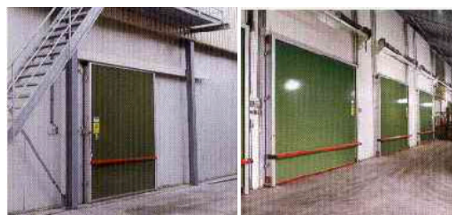
Fig. 1: The left, pictured shows the Doors may be fixed on a sliding rail, and the right side picture shows the mounted to open vertically on overhead rails.
