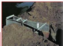
A Parshall - type flume.
