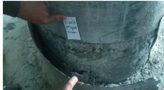
Figure 2: Spalling of concrete at the 2nd cycle of 1% drift
