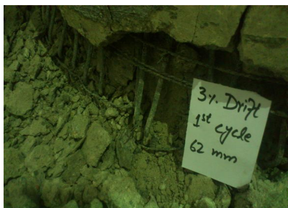
Figure 4: Ruptured bars at 3% drift
