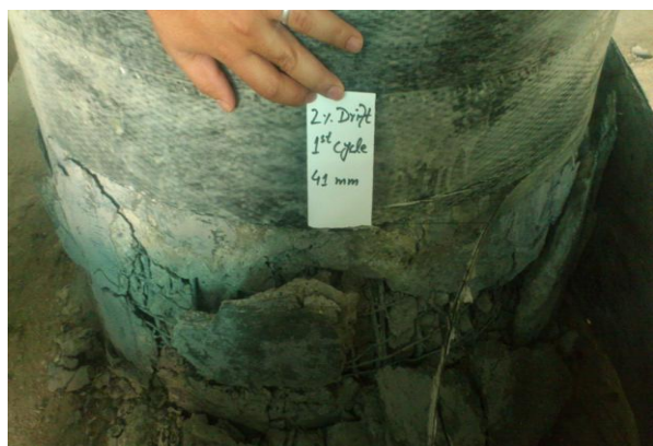
Figure 3: Spalling of concrete and buckling of rebars at 2% drift
