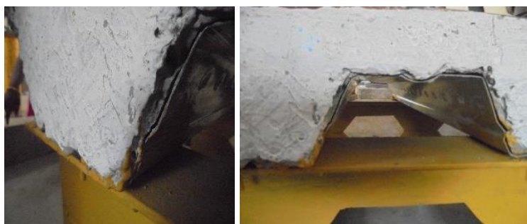
Figure 5.3 Delamination of Profiled sheet
