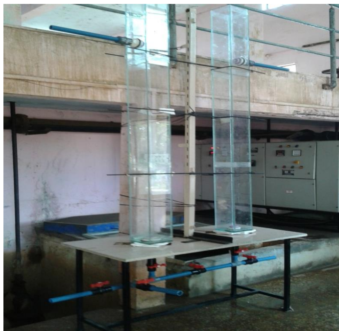
Figure 2 Installed pilot plant at Ichalkaranji W.T.P
