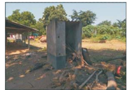
Fig 10: Public Latrine (Abandoned), Amkopa
