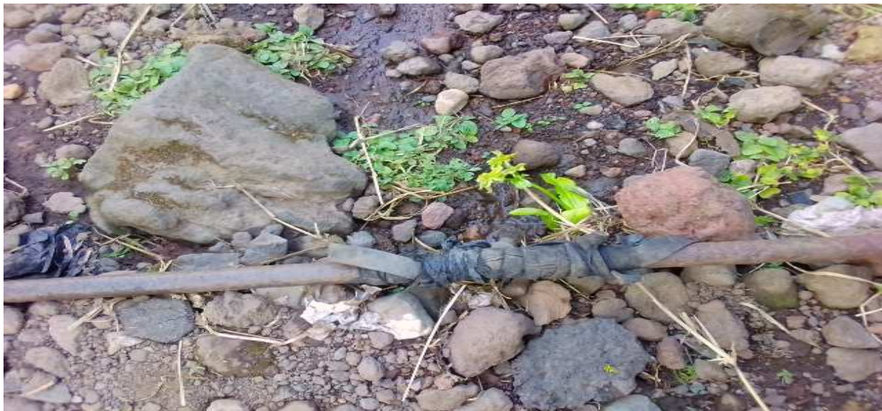
Figure4; An exposed and broken locally patched pipe leading to households
