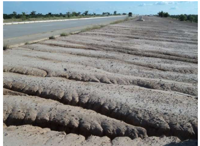
Figure 2 Channel and Piping Erosion
