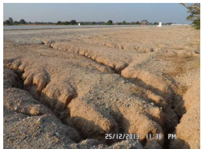
Figure 3 Channel and Piping Erosion
