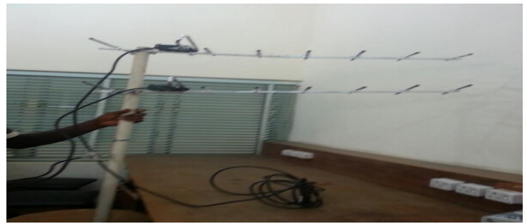
Figure 2: Vertical dual-stacked antenna
