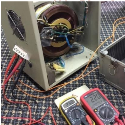
Figure 11. Photo showing 7kVA, Automatic Voltage Stabilizer Control System at over-voltage Condition
