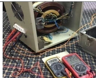
Figure 9. Photo showing 7kVA, Automatic Voltage Stabilizer Control System at Normal Condition
